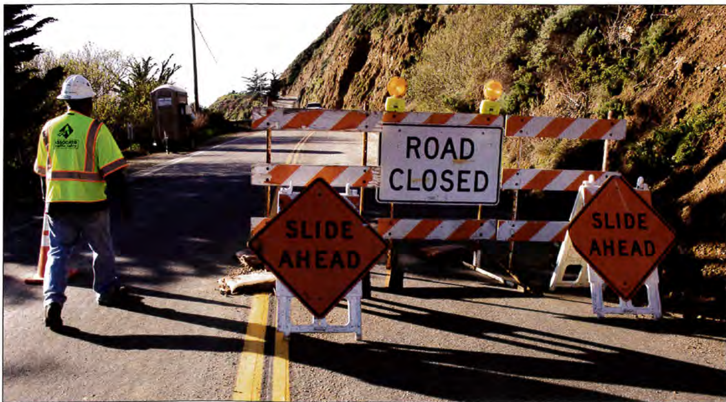
After major wildfires and subsequent heavy rains, the Pfeiffer Canyon Bridge in Big Sur collapsed from a slide and had to be replaced. From March to October, 2017, access to Big Sur was severely restricted.
